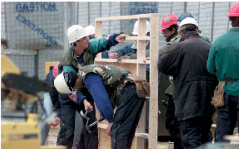
Bosnian civilians employed by a US military contractor work on a construction project during Operation JOINT FORGE.
